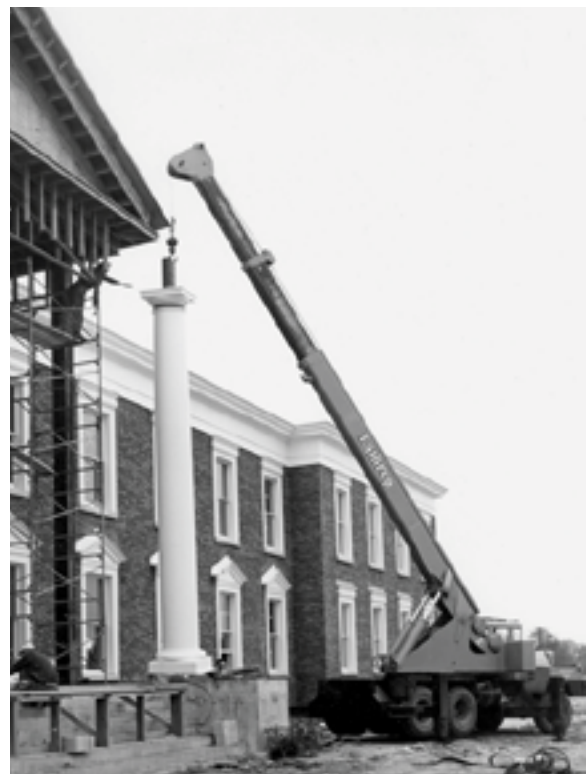
Dana's headquarters moved from the Bennett Road production complex in Toledo to 4500 Dorr Street in 1970. At the same time the building was going up, Chairman Jack Martin and President Ren McPherson were flattening Dana's management structure to strengthen the company's competitiveness.
